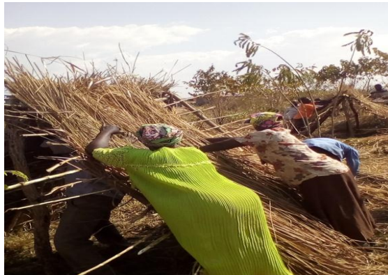
Women building their own makeshift houses on their pieces of land at Kyakaboga resettlement site.
